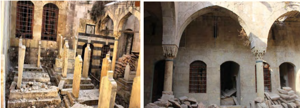
Figure 4, Damages done to portico (Al-Ahmadiyya school in Aleppo article)
